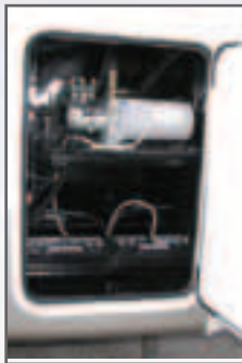
Challenger's dual battery and hydraulic pump utility compartment. (Batteries not included)
