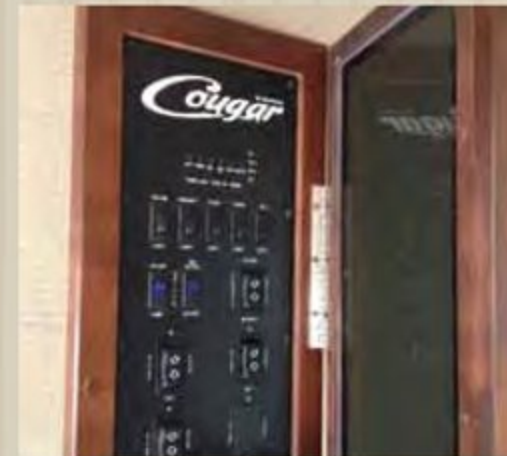
Cougars command center features backlit switches and places all of your controls in one convenient location.
