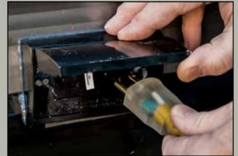
Convenient Outside GFCI Protected and Covered Outlet.
