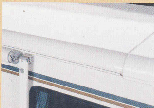
1-YEAR OLD ITASCA FIBERGLASS ROOF
