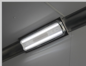
24" LED INTERIOR LIGHTING.
