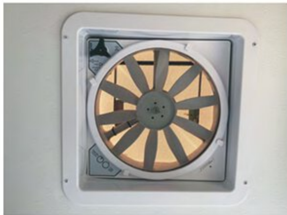
High Output Attic Fan in Bathroom
