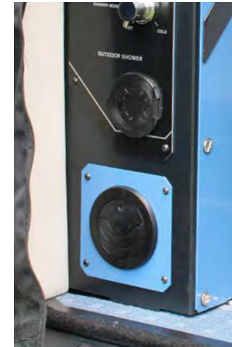
Upgraded Rixen Hydronic System with 2 Blowers
