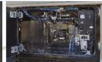
Easy access water bay and 50 amp power land line
