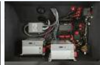
Deutsch heavy-duty, water-tight, bulk connectors with two 3,000 watt power inverters shown
